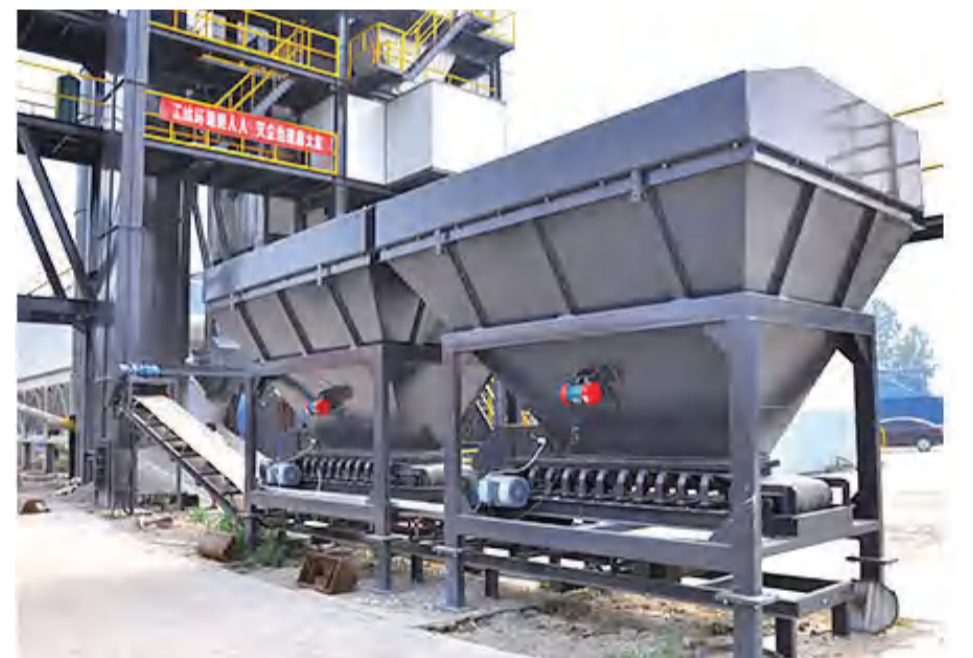
(RAP)Recycle/ Reclaimed Asphalt Plant in Peru
