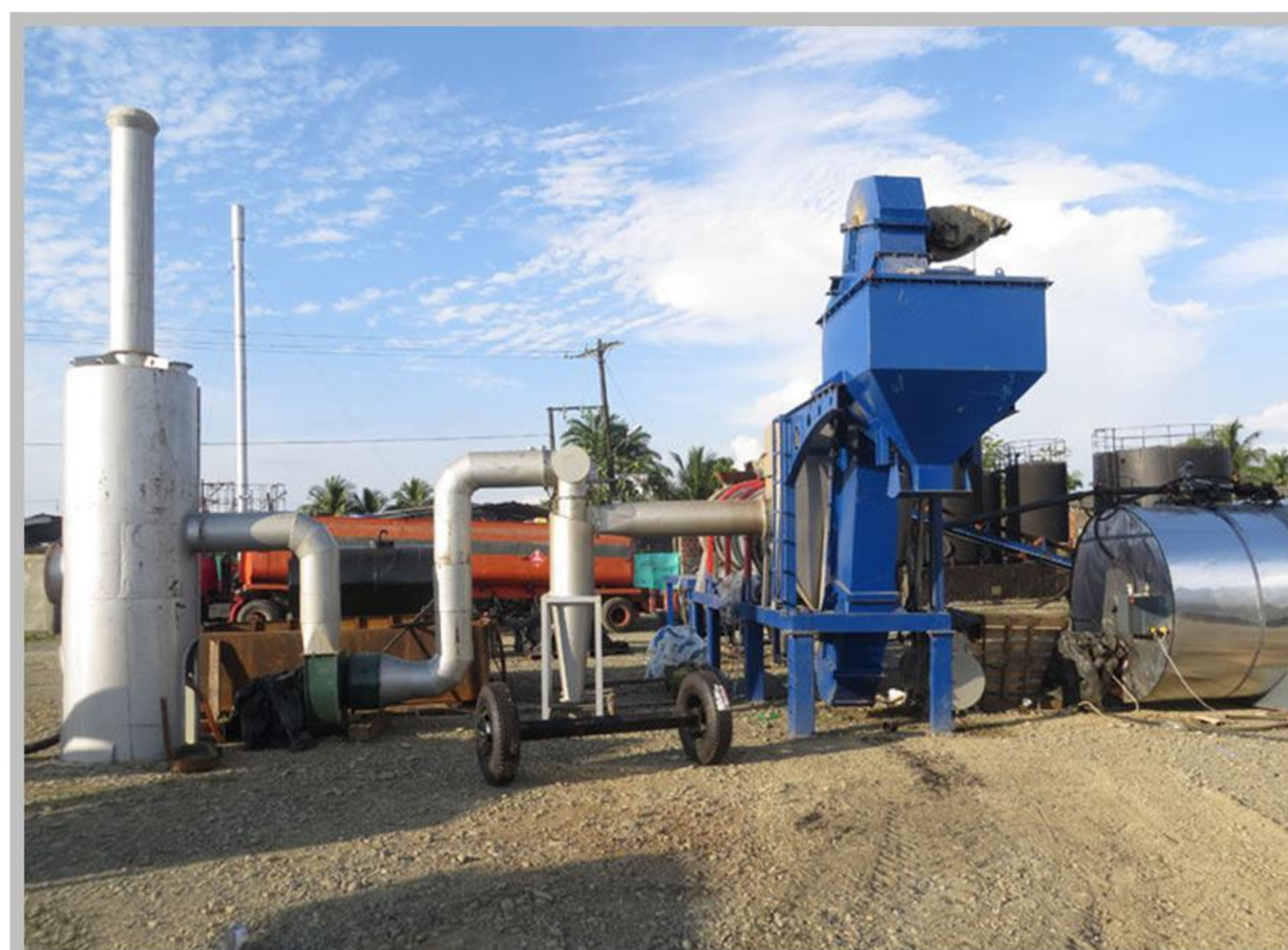
continuous asphalt mixing plant in Ethiopia
